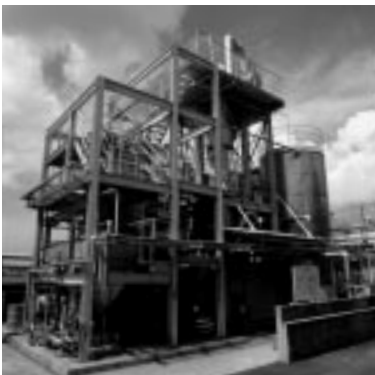
Evaporator of Shochu Waste at the Moji Plant
