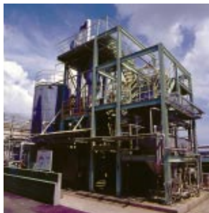
Concentration plant for shochu distillate
