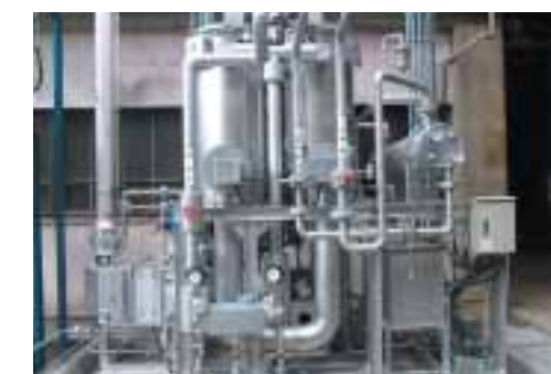
Xylene recovery equipment
