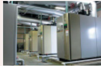
Boiler fuel conversion at the Fuji Plant (completed in November 2005)
