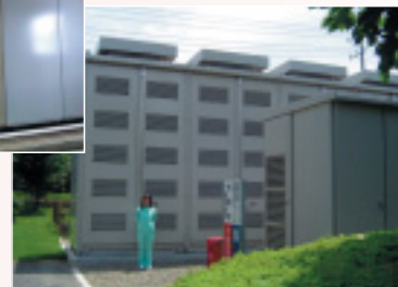
The NAS battery system at the Kyowa Hakko Food Specialties Tsuchiura Plant (installed in May 2006)
