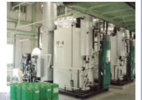
▲ Gas boilers at the Hofu Plant
