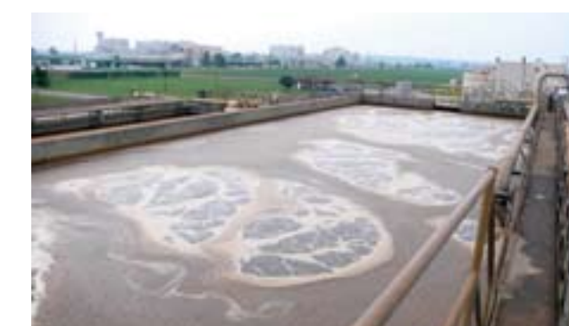
A wastewater treatment tank
