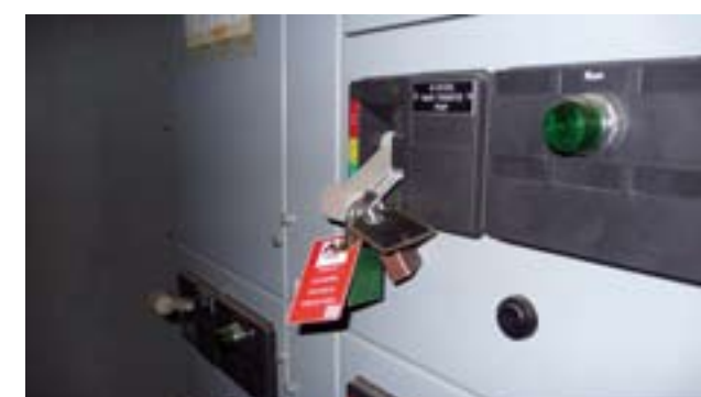
Machinery lockouts (attention to safety)
