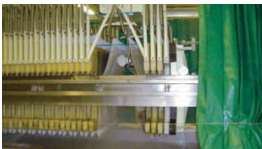
A phosphoric acid recovery facility dehydrator
