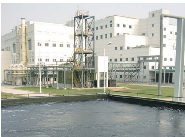
A liquid-waste treatment facility
