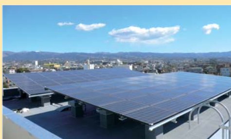
Photovoltaic power generation system
