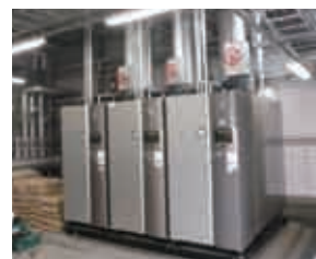
The boiler relocated to near the research facilities
