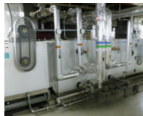
New air handling unit
